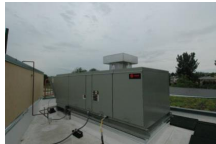
High Efficiency HVAC
