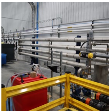
Wastewater heat recovery
