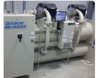
Two new 250-ton Magnetic Oil-free Centrifugal Chillers with variable frequency drives
